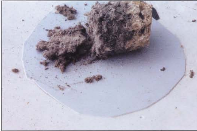
Core cuts show dry insulation.
