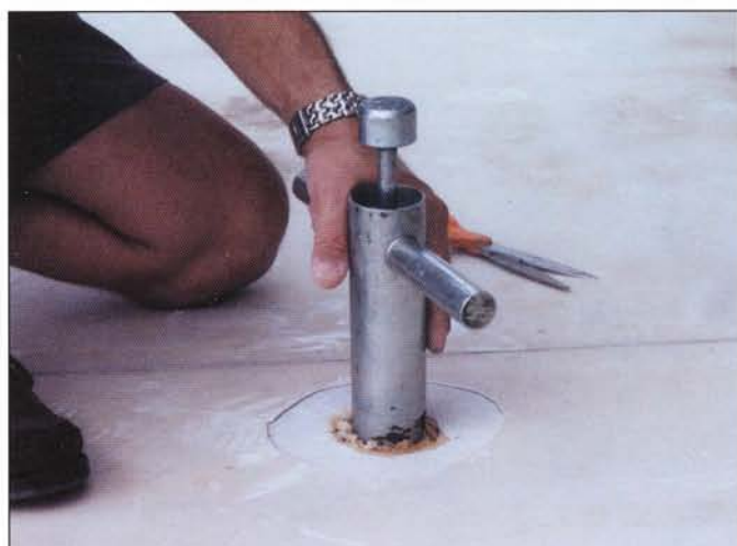
Core cuts were made in two of the previously identified wet areas.
