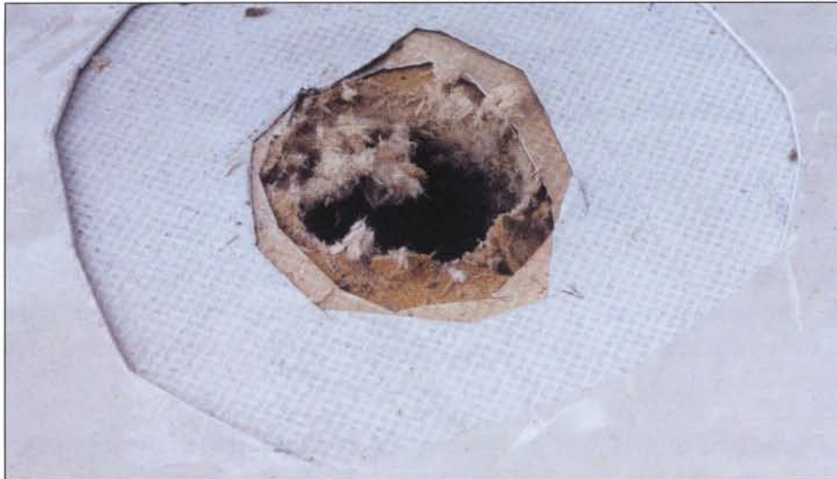
Cuts were made through the new membrane, existing Hypalon membrane and insulation, down to the vapor barrier.
